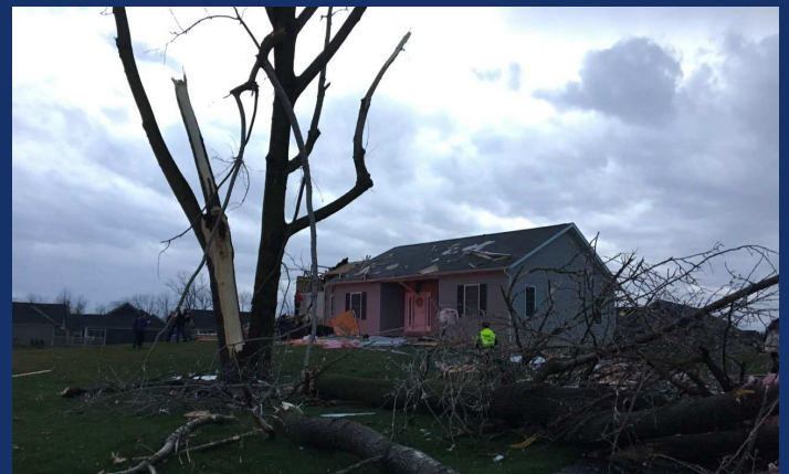
Grove City Tornado Damage
